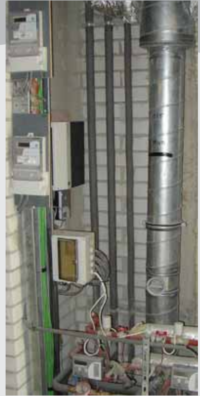
All meters are located in central, vertical ducts
